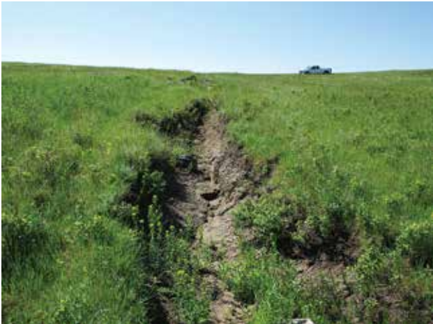
Gully with some active side and bed cutting and some vegetation on sides and bottom.
