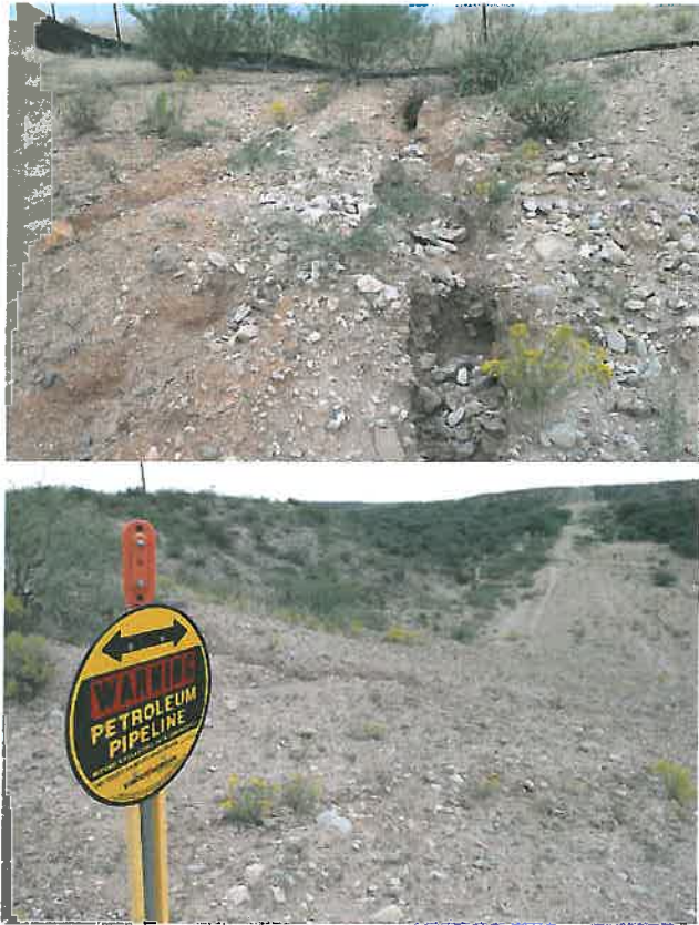
Figure 1. Views of the Kinder Morgan pipeline near Cienega Creek. Constructed in 2007, erosion (top) and slow to no regrowth of vegetation (bottom) are evident in these photographs, which were taken in 2013.
