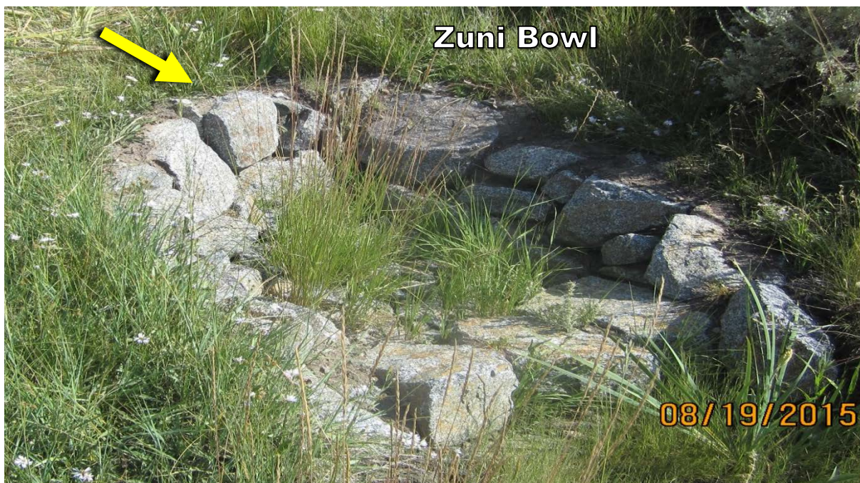
Figure 7. It is critical to ensure the top rocks of the Zuni bowl wall match the existing elevation of the headcut pour-over (denoted by yellow arrow). This helps irrigate vegetation at the lip, allowing it to become the most vigorous instead of the weakest point subject to erosion. If rocks are too high, they divert water around structure, concentrate flow, and potentially cause new gullies. If rocks are too low, soils and roots are exposed and vegetation dies. Photo by: Nathan Seward
