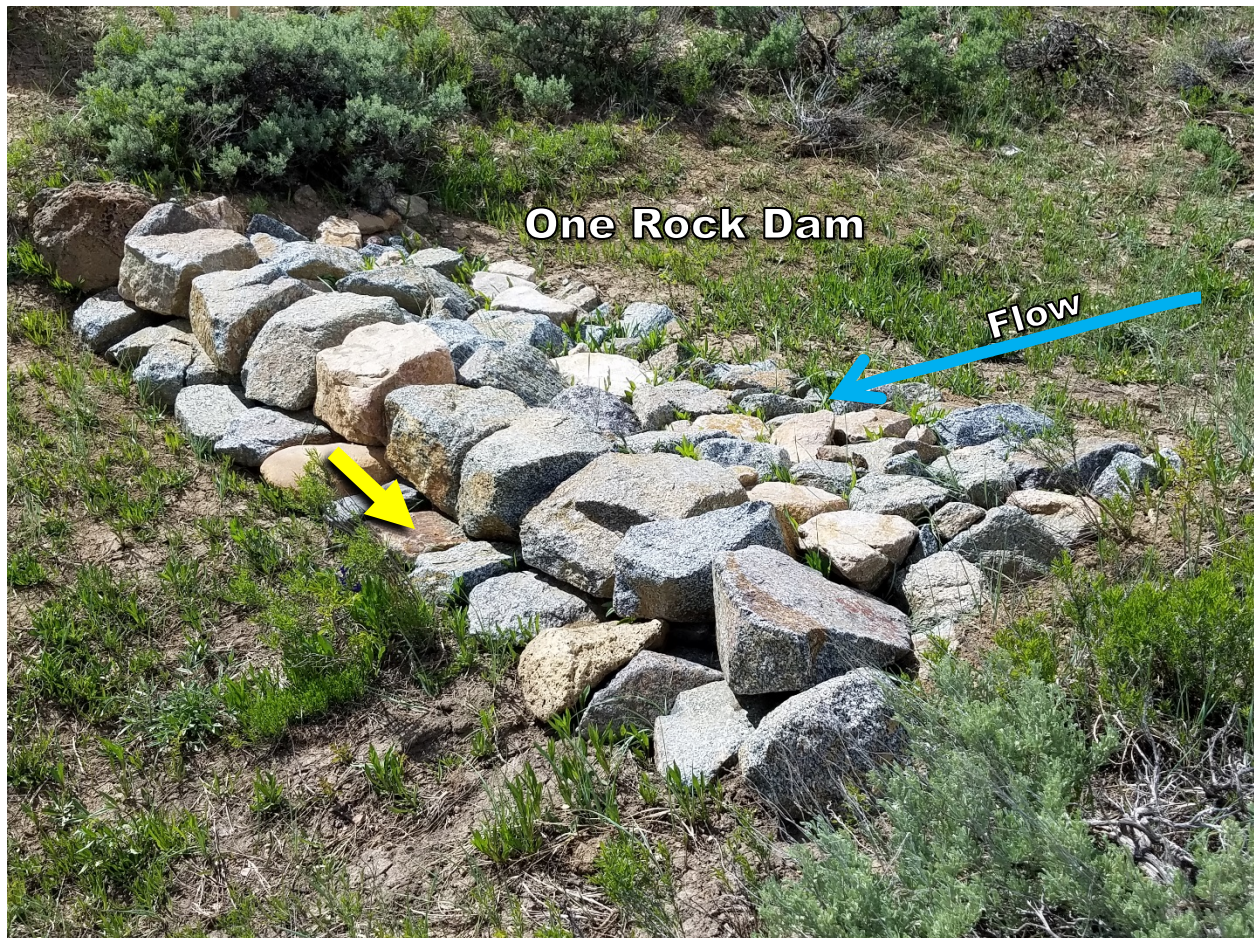
Figure 14. One rock dams should have a footer for splash apron on the downstream end that extends far enough to intercept water pouring over the structure in a high flow event (denoted by yellow arrow). Photo by: Nathan Seward
