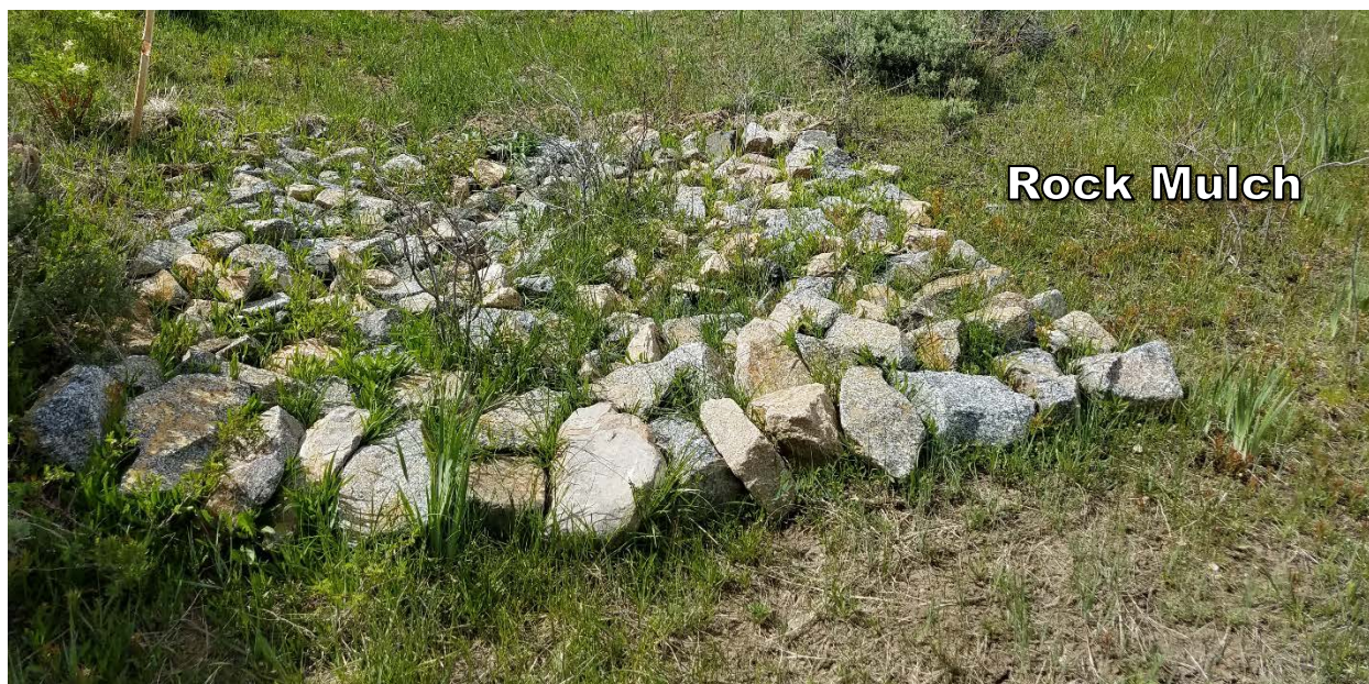
Figure 11. Rock mulch can be used in off-channel areas to address minor headcuts and return flow sites. Photo by: Nathan Seward
