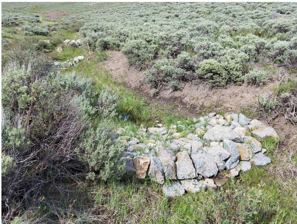
Zeedyk rock structures installed to restore incised channel. Photo by: Nathan Seward
