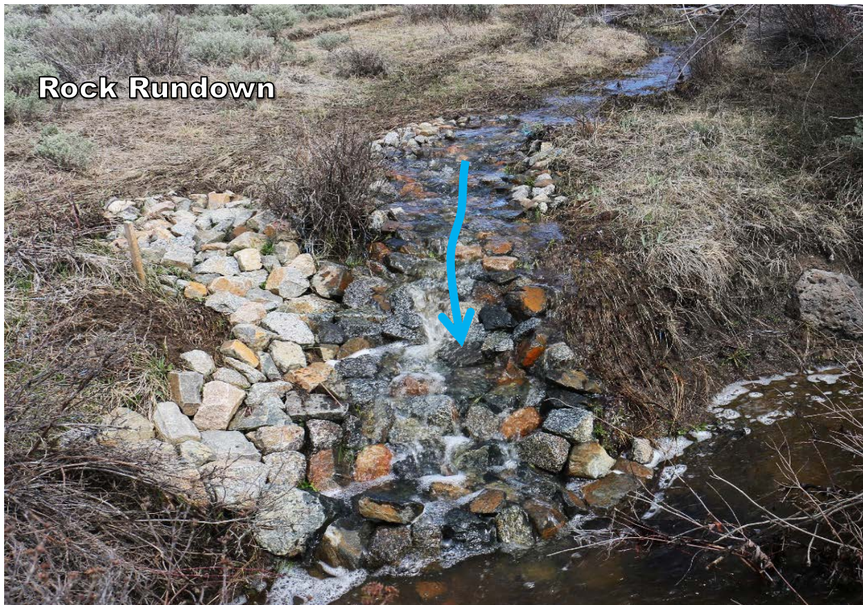
Figure 10. The center of a rock rundown should be the lowest so water runs down the middle and not around the structure. Photo by: Nathan Seward
