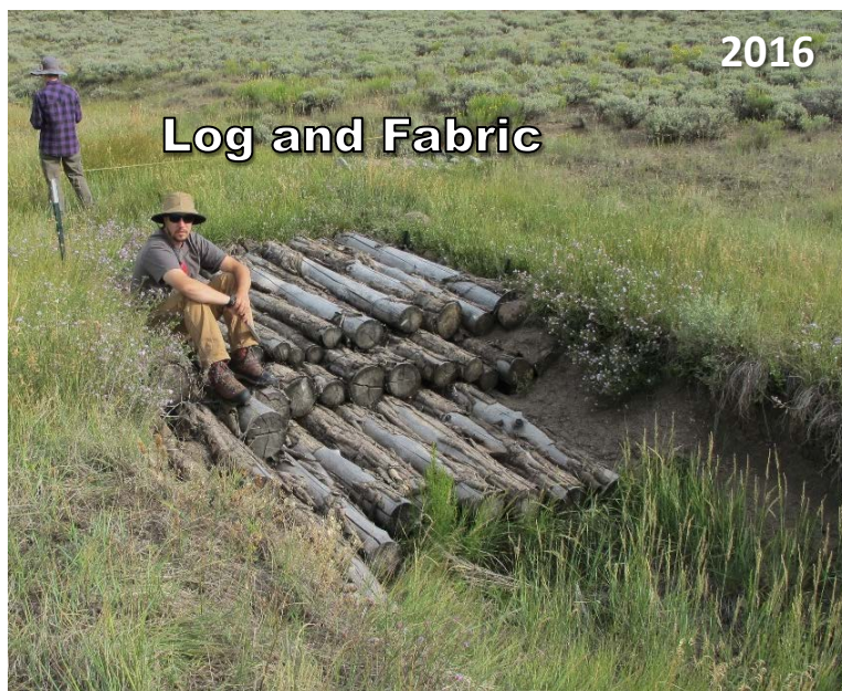
Figure 13. Log and fabric structure for treating headcuts before (top) and after (bottom) installation. Photos by: Renee Rondeau
