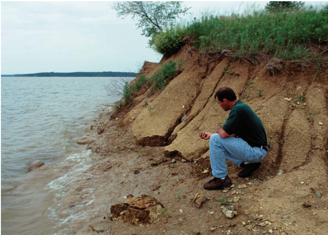
Figure 600-B5: Soil erosion – excessive bank erosion from stream, shorelines or water conveyance
