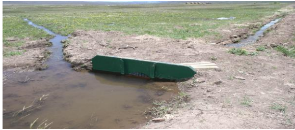
Fig. 5. Example of a headgate used for diverting water in a mountain meadow. Differing numbers of board slats are placed in the slot on the face of the structure to control how much water flows into each of the ditches. (Photo by John Scott)
